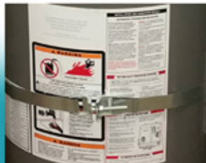
WATER HEATER SEISMIC STRAPPING
